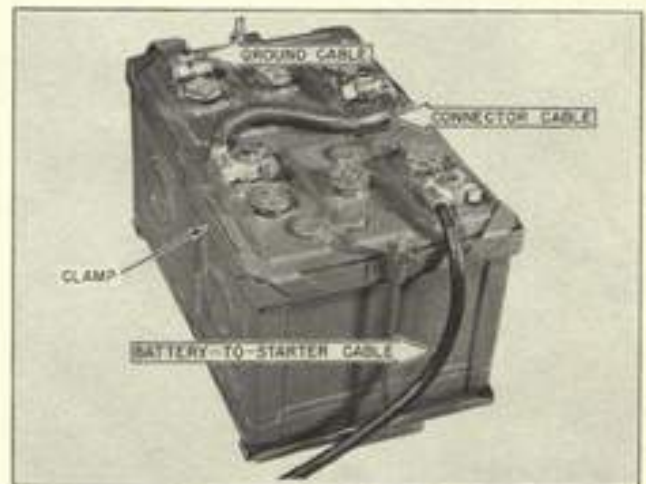
Figure 4-5 Batteries Connected For Diesel Installation
