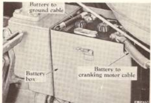
Illustr. 65 Battery and cables.
