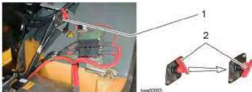
Switching the battery main switch on and off
