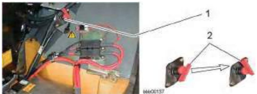
Battery main switch
