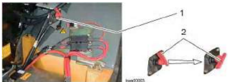
Turning off the battery main switch
