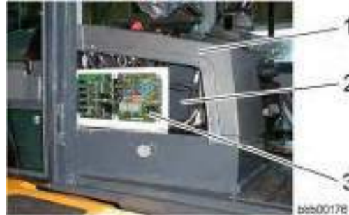
Fuse box with A4 control board
