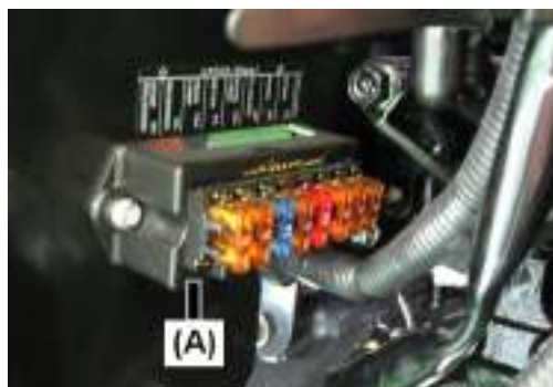
(A) Fuse box
