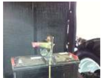
Fig. 3-26 Main power switch
