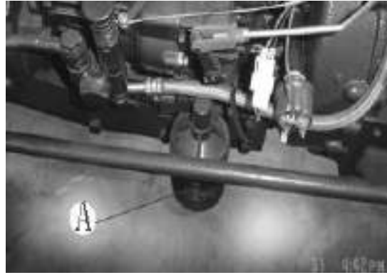
Figure 4-25 Engine Oil Filter Maintenance
